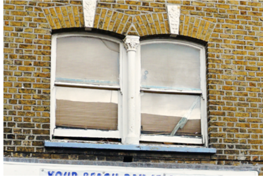
Joinery in poor decorative condition on the High Street
