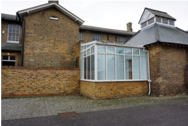
Inappropriate uPVC conservatory to the rear of one of the barracks blocks
