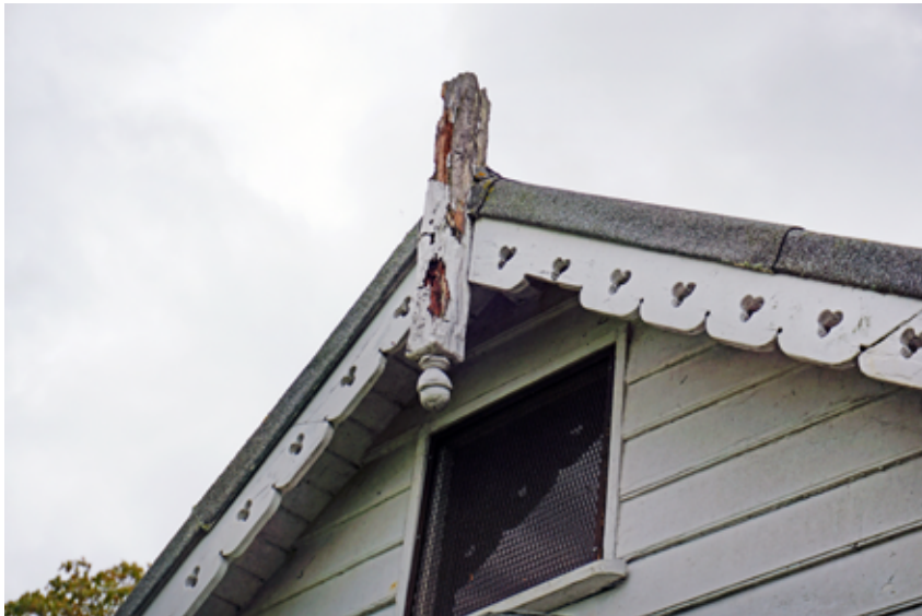
Deteriorating woodwork on the cricket pavilion
