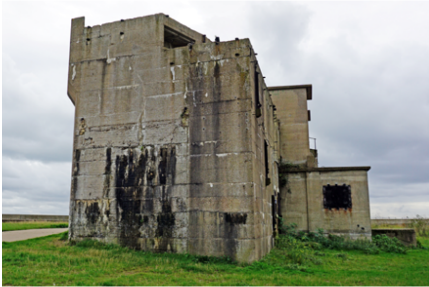
Salt and water staining, and cracked concrete to the Heavy Quick Firing Battery (some remedial work has been carried out to this structure)
